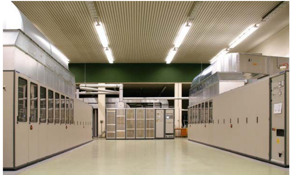
800 kW transmitter TRAM/P800 756kHz
