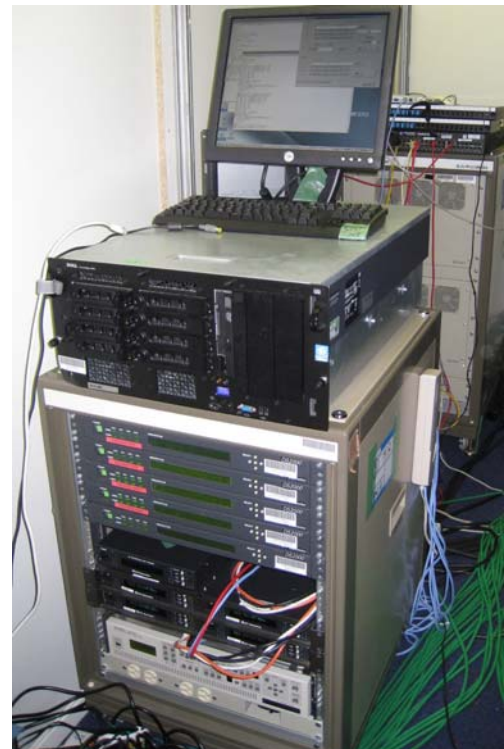
Figure 3 Receiving equipment at the SHV Theatre
