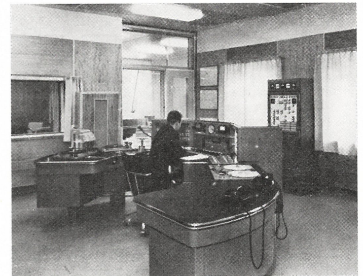
Fig. 7. — Continuity suite fully adapted for stereophony in service in the V.A.R.A. studio-centre at Hilversum.
